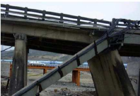
Figure 1 Damage to Communication Backhauls due to Earthquake
